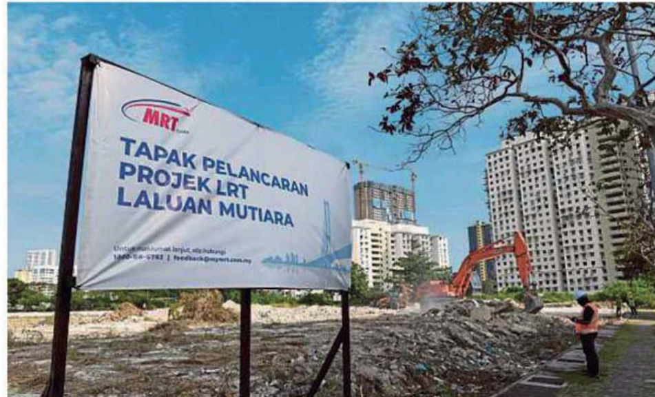
The site of the Penang Light Rail Transit project being prepared at Lebuhraya Pinang last Friday.
